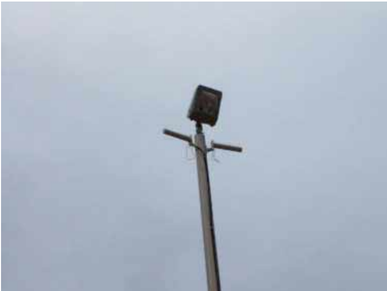
Figure 52 Yagi Antennas for wireless backbone
