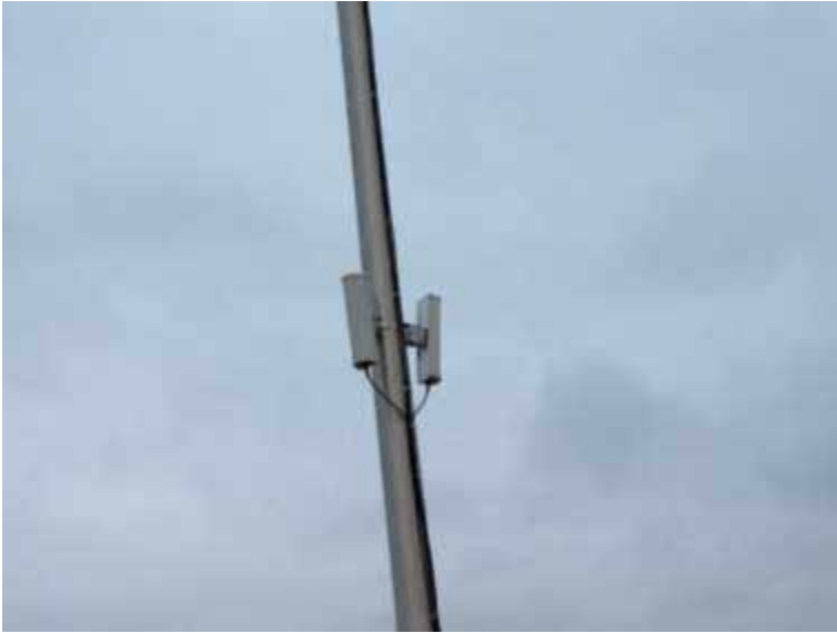
Figure 13 Sector Antennas for AP coverage
